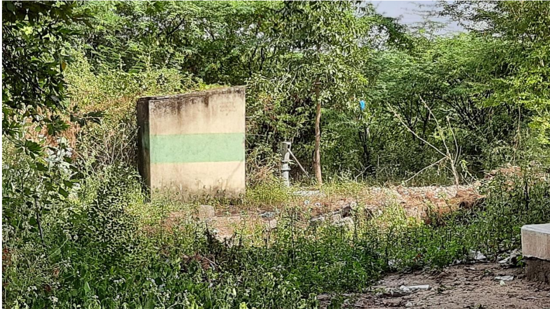
c) KOOVALAPURAM MUTTUTHURAI RESTROOM AND WATER PUMP WITH NO WATER FACILITIES
